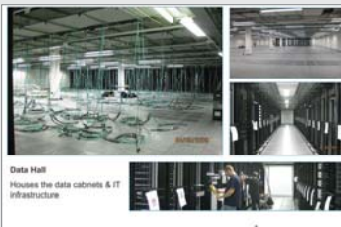
The Ground Floor hosts all electrical and mechanical infrastructure necessary to support the data halls located on the Mezzanine level.
